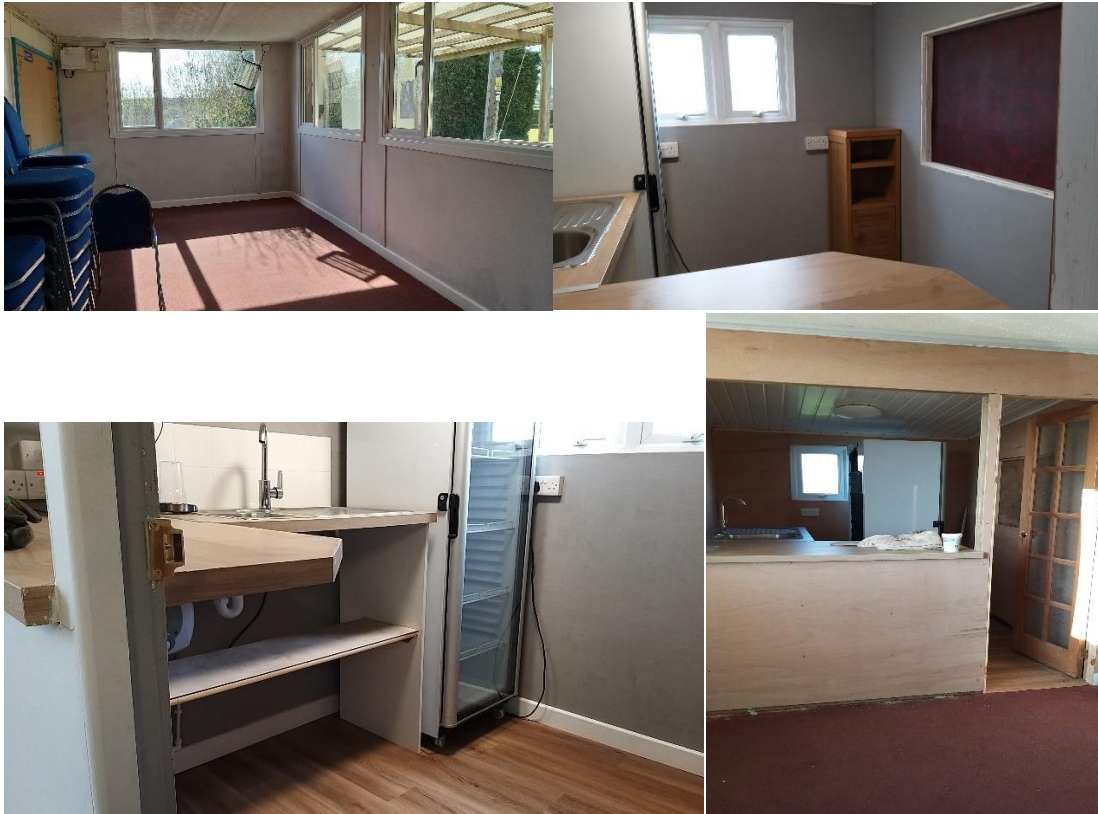
Figure 4 Last summer's outside area with gazebos, new covered structure evolving that will provide a more resilient framework and support sail coverings
